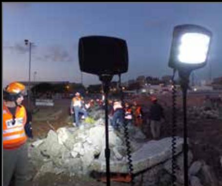
Ideal for emergency power in natural disasters
